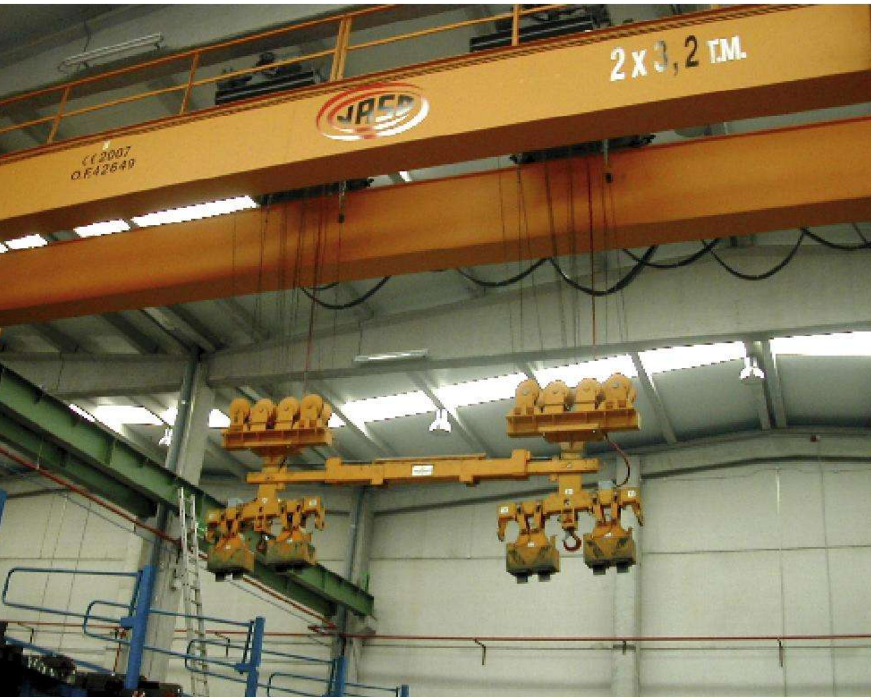
STORAGE E.O.T. CRANE 2X3,2 T - 21.35 M SPAN.
