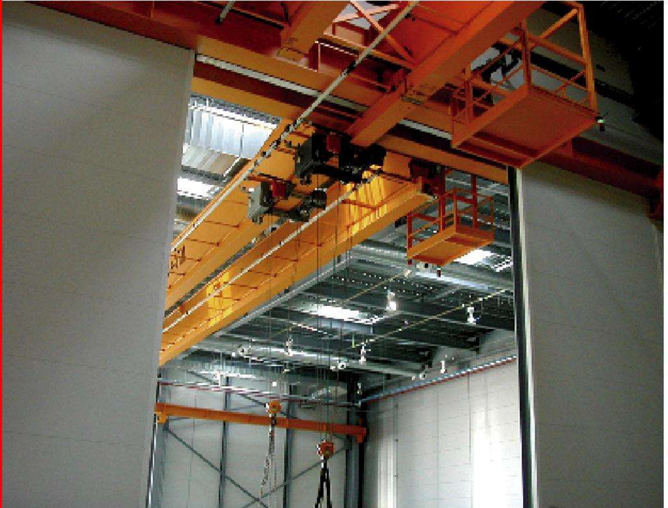
TRANSFER E.O.T. CRANE 5+5 T - 38.49 M SPAN.
