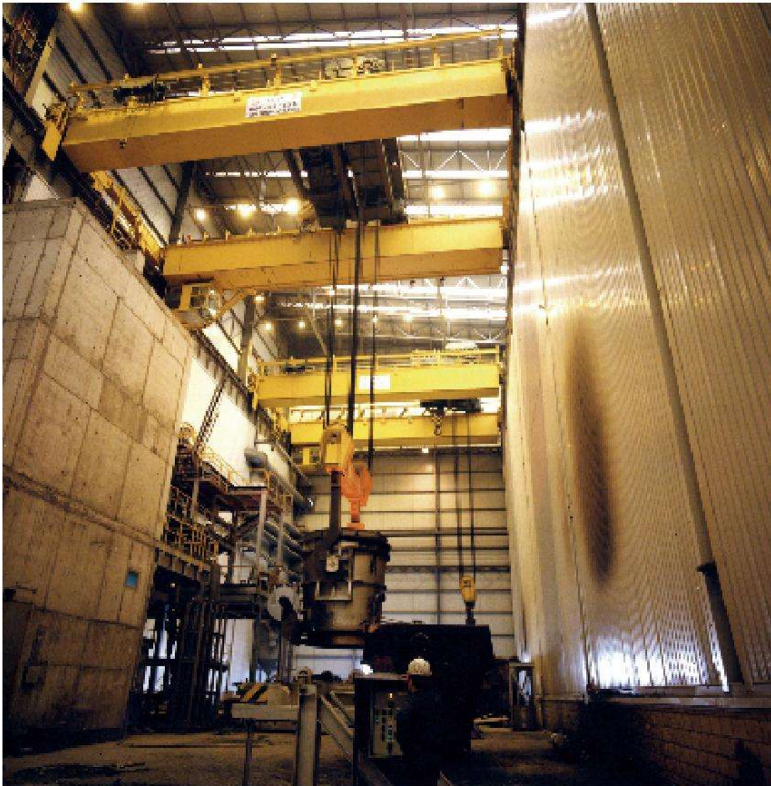
LADLE E.O.T. CRANE 220/63/10 T - 25 M SPAN.
