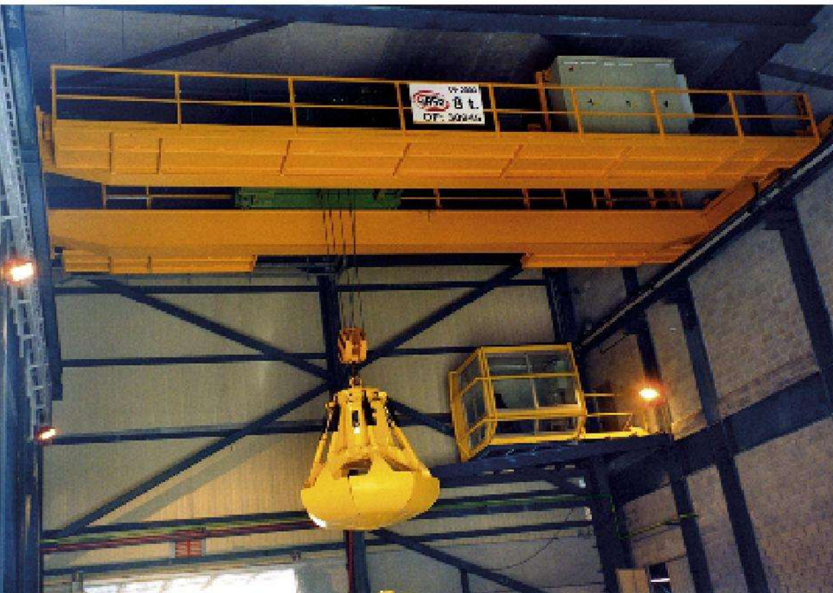
WASTE TREATMENT E.O.T. CRANE 8 T - 15 M SPAN.
